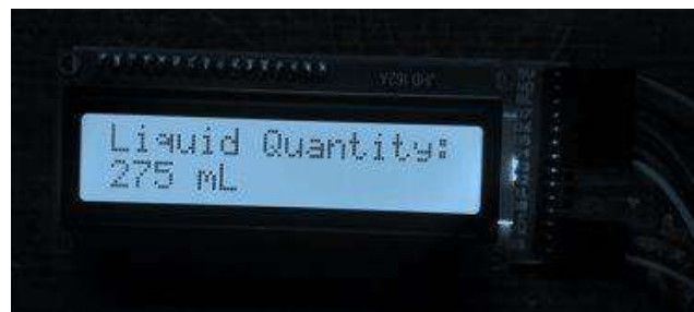
Fig. 7. Flow Meter Screen Notification
